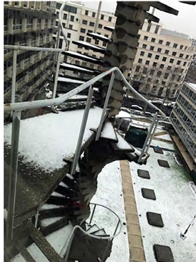
A precarious-looking exit stair (no longer the primary means of emergency egress) at Breuer, Nervi, and Zehruss' UNESCO Headquarters Paris, 1958; photograph by the author, January 2019.
