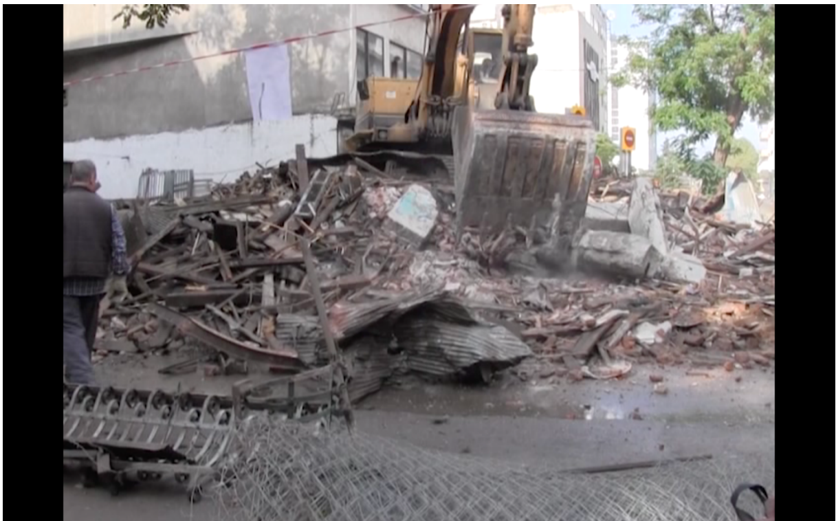
25. Vardaris, house demolition 2015 to broaden the street for a parking lot. Video stills from Outtakes 2 , produced in the realm of the exhibition; we can never fly first class , Munich City Museum, Gallery Einwand, 2023.
