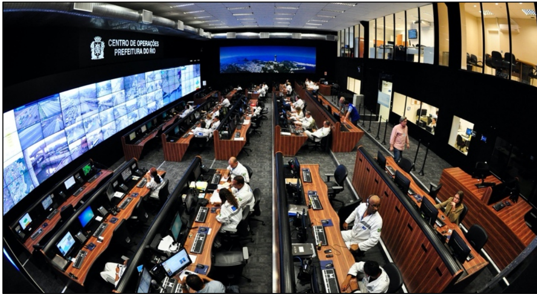
Fig. 19—Rio Operations Center, Rio De Janeiro, 2014. (Source: IBM News Room)
