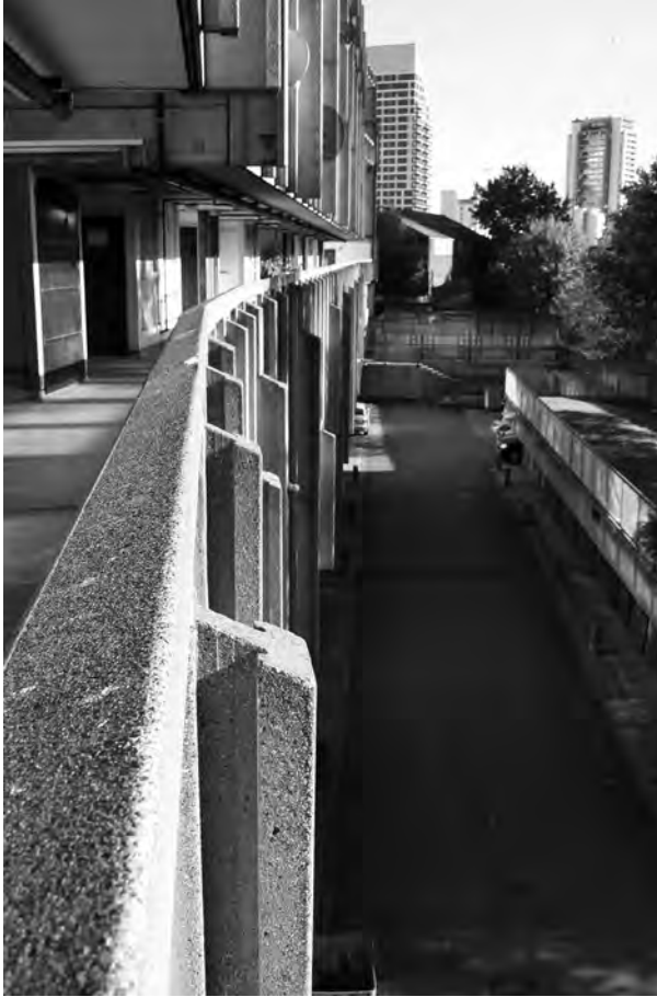
Figure 6.6 Over the edge of a street deck on the west block, showing the balustrade, mullions and garage moat. (Nicholas Thoburn, September 2015)
